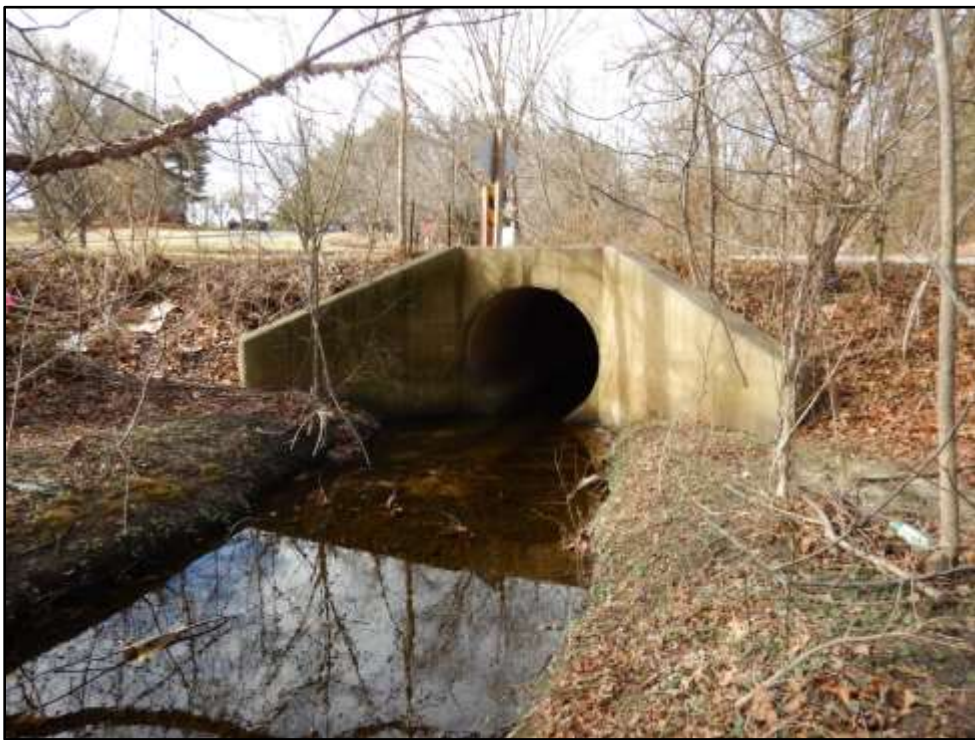
Photo 10: Looking at the downstream side of the Little Plumtree Branch crossing at the private driveway entrance to Resurrection St. Paul School. Photo taken January 18, 2017.
