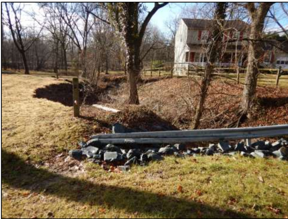
Photo 4: Looking downstream at erosion along Plumtree Branch from Longview Drive. Photo taken January 18, 2017.
