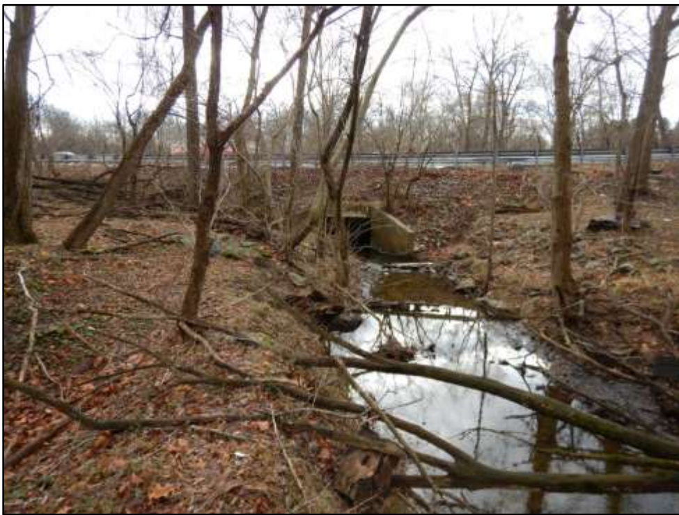
Photo 2: Looking toward the upstream side of the Plumtree and Rt 40 crossing. Photo taken January 18, 2017.
