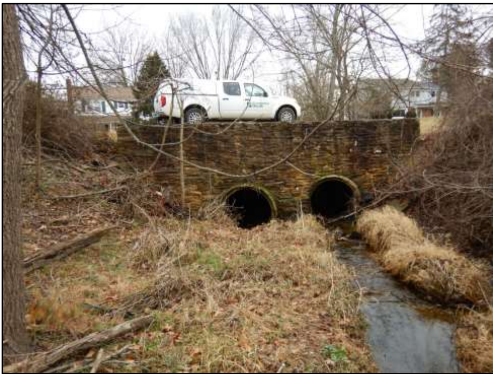
Photo 8: Looking at the upstream side of the Plumtree Branch crossing at Hearthstone Road. Photo taken January 18, 2017.
