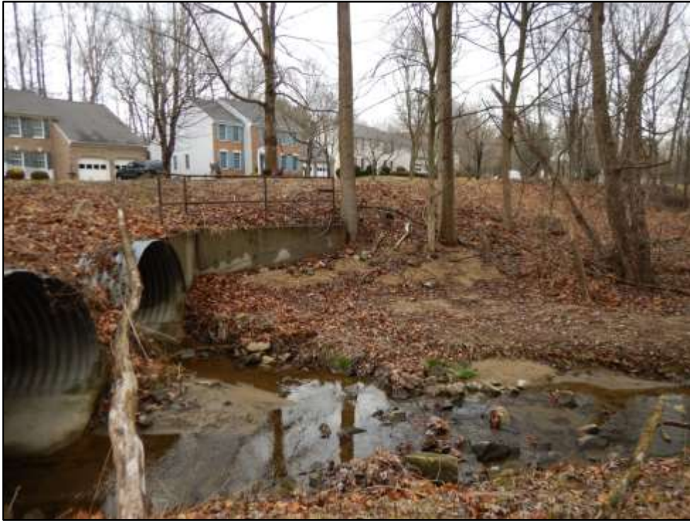
Photo 9: Looking at the downstream side of the Little Plumtree Branch crossing at Michaels Way. Photo taken January 18, 2017.
