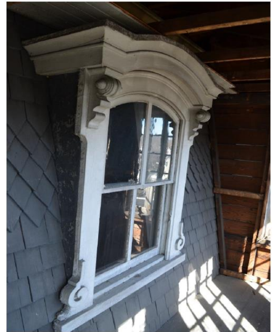
Figure 12 – Photo from application - Mansard roof and window currently covered by second floor porch enclosure.
